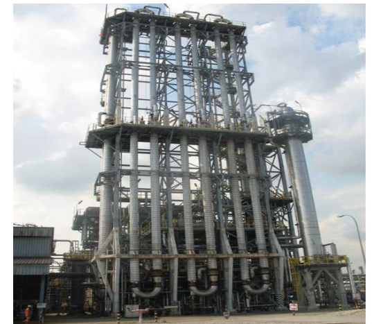
The modern oxo alcohol reactor in Singapore (on the far right) has the same reactor volume as four large loop reactors combined (to the left), but with a much smaller footprint.
